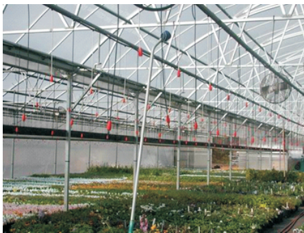
Hose nozzle hung in greenhouse
